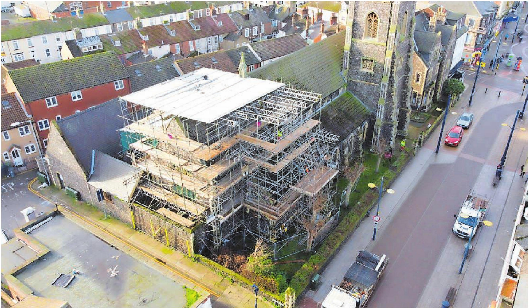
Drone pictures offering a bird's eye view of urgent restoration work going on at St Mary's RC Church in Regent Road, Great Yarmouth, and its place in the town
