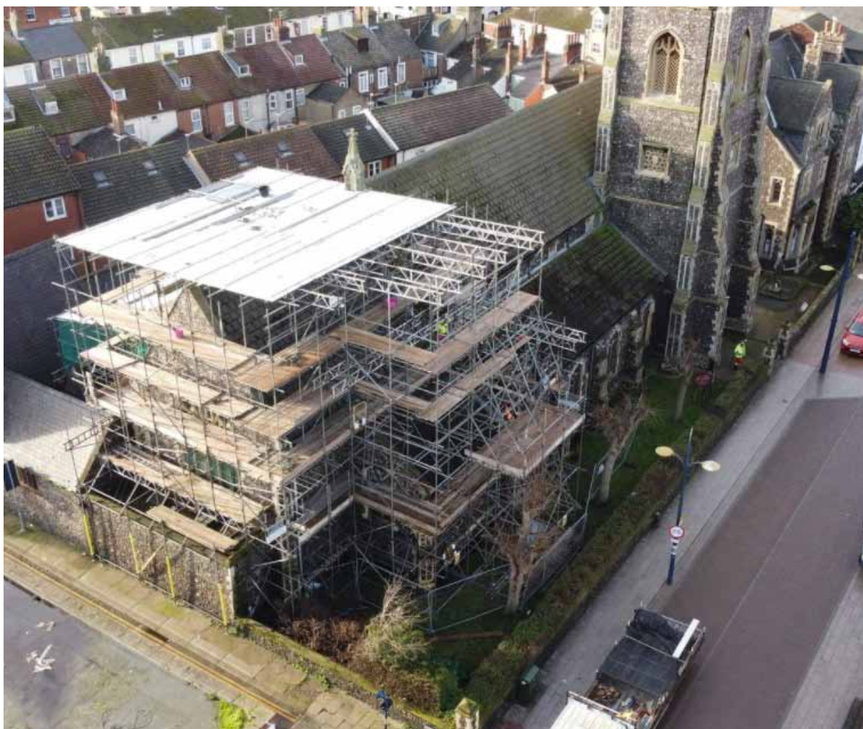
Drone pictures offering a bird's eye view of urgent restoration work going on at St Mary's RC Church in Regent Road, Great Yarmouth, and its place in the town
